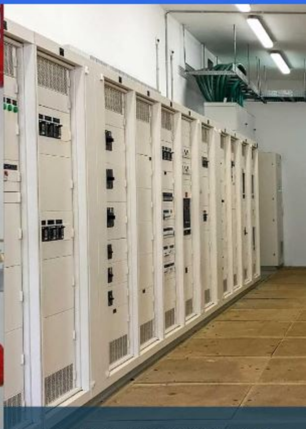
POWER, LIGHTING AND ICT
